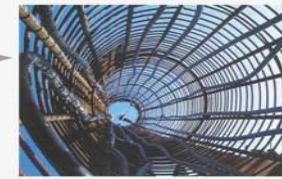
Earth pipes in pile foundation provide together with heat pumps heating and cooling throughout the year
