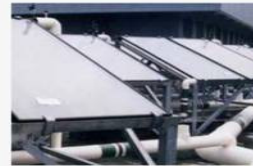
Solar water heating panels on roof area greatly reduce overall water heating load
